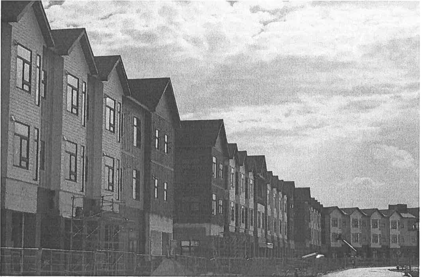
The Willoughby Corner housing project is pictured under construction on July 16, 2024, in Lafayette. (Andy Colwell, Special to The Colorado Sun)
